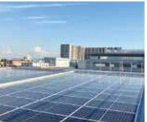
Rooftop solar panels
